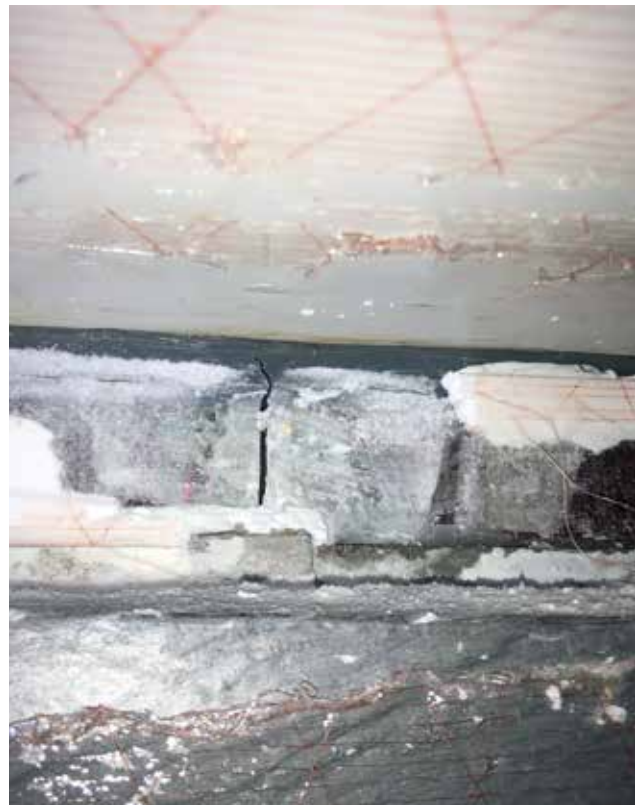
Fig. 1) Crack at the Mastic line
