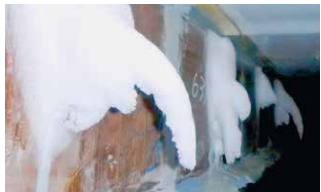
Fig. 2) Cold spots in supporting system
